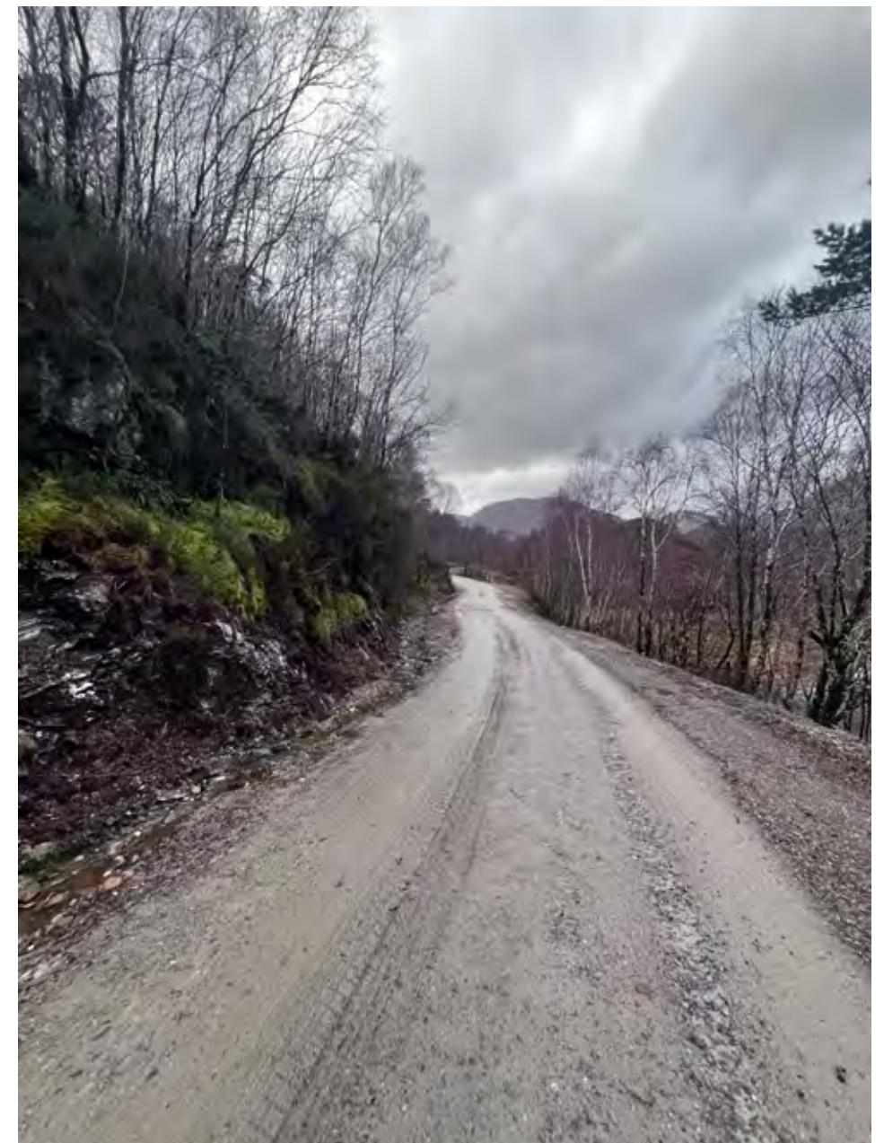
Steep rocky cut / steep slopes either side of track
